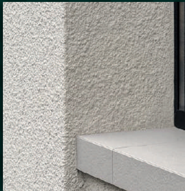
3 - PLASTER WITH PAINT
